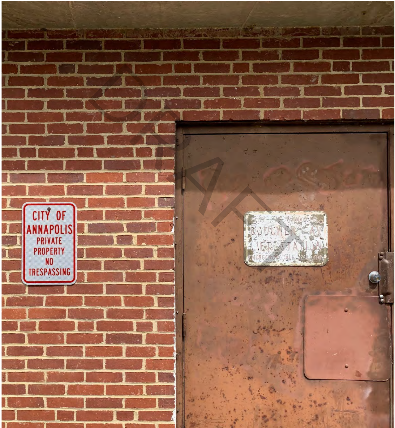
FIGURE 10-18: (LEFT) THE CITY'S BOUCHER AVENUE LIFT STATION LOCATED AT HAWKINS COVE IS ONE OF MANY SMALL BRICK STRUCTURES LOCATED THROUGHOUT THE CITY THAT HOUSE PUMPS FOR MOVING WASTEWATER FROM LOWER TO HIGHER ELEVATIONS.
