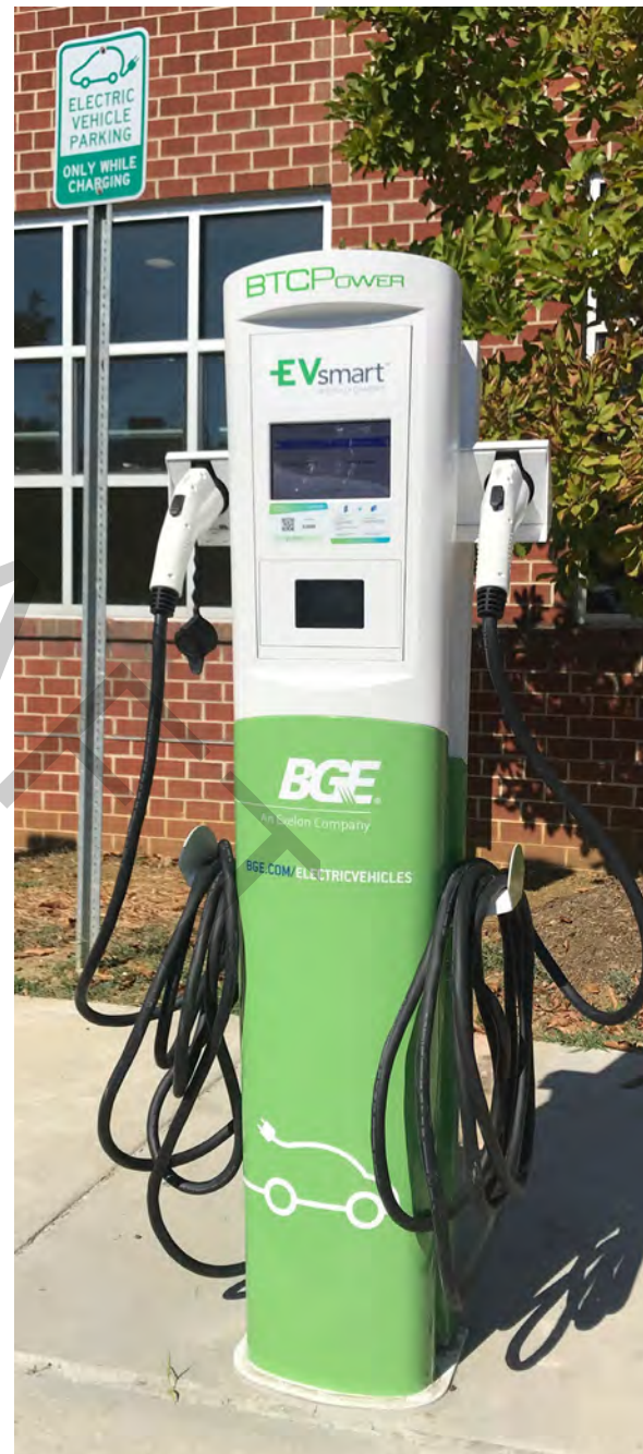
FIGURE 9-28: EV CHARGER AT PIP MOYER RECREATION CENTER
