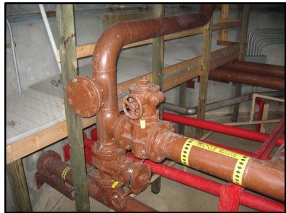
Lines at the Sewer Treatment Plant
