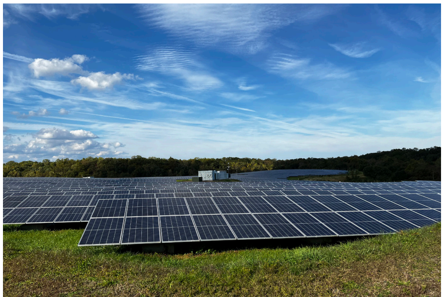
The Annapolis Solar Park, constructed on a brownfield site at the former Annapolis City Landfill.
