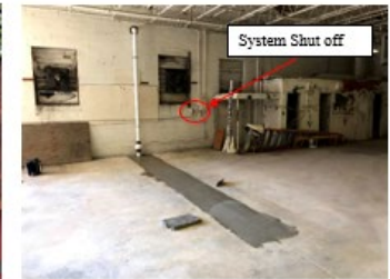
Photograph 2. PRIMARY SYSTEM – Fan and Connections Fan should be running, there should be no loose connections and black bolt or lock which prevents shut off should be present
