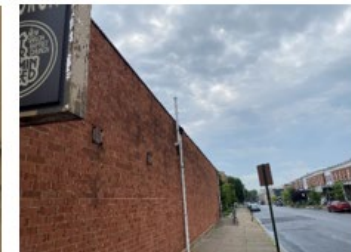
Photograph 4. SECONDARY SYSTEM Exterior View – Vapor Mitigation System Exhaust Piping Vent should be free and clear of obstructions
