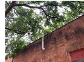
Photograph 1. PRIMARY SYSTEM Exterior View – Vapor Mitigation System Exhaust Piping Vent should be free and clear of obstructions
