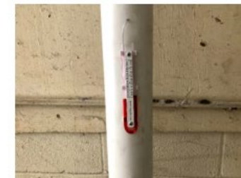
Photograph 3. PRIMARY SYSTEM – Vapor Mitigation System Gauge Gauge should show a pressure difference between subsurface and outside air (as shown)
