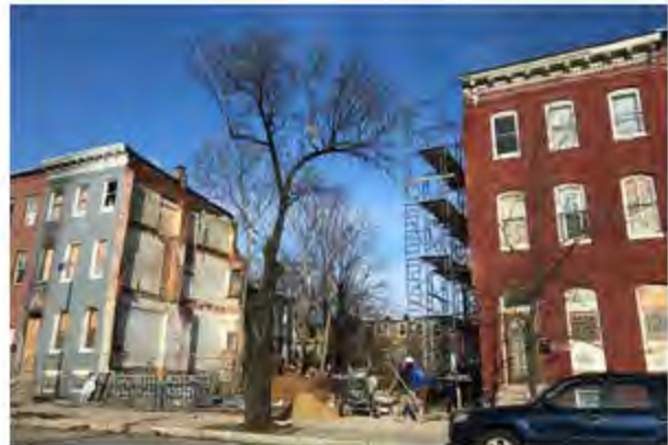
Demolition site next to a vacant rowhouse, northwest corner of Wilkens Ave. and Monroe St.
