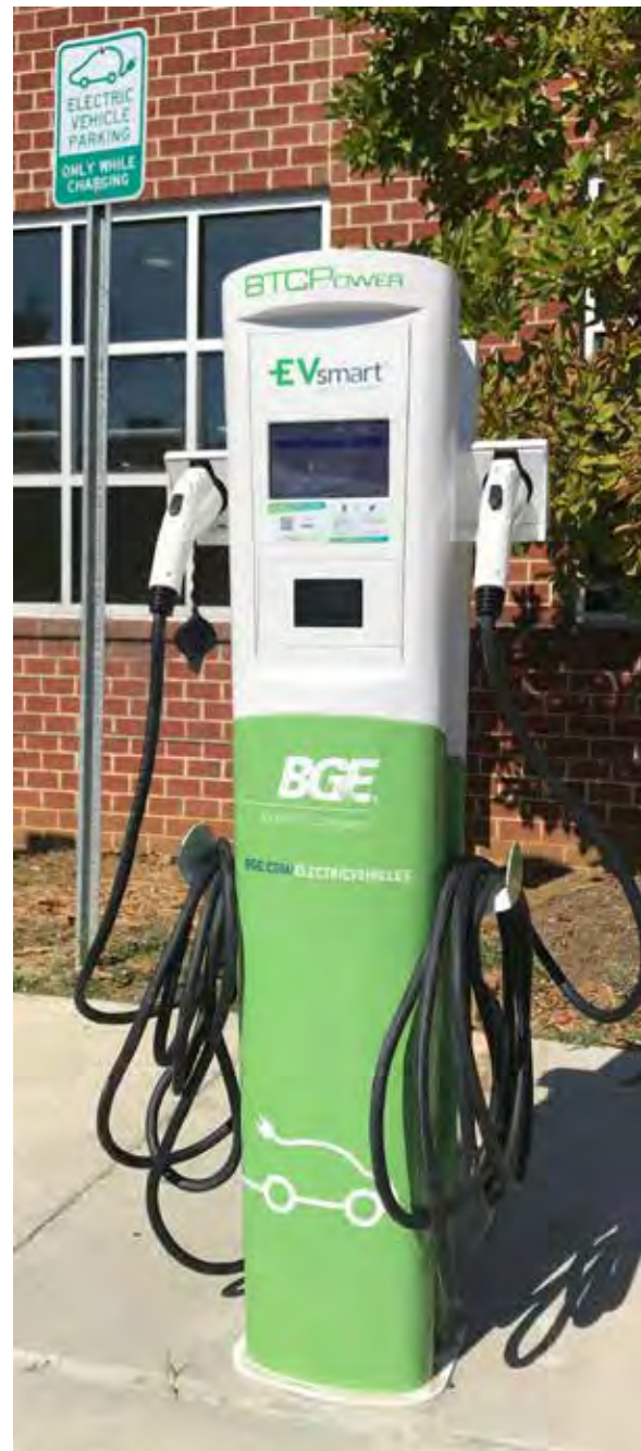
FIGURE 9-28: EV CHARGER AT PIP MOYER RECREATION CENTER
