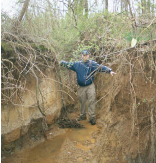
Figure 4 Excessive stream bank erosion and channel downcutting along a tributary of the Muddy Branch creates a high priority stream restoration candidate site.
