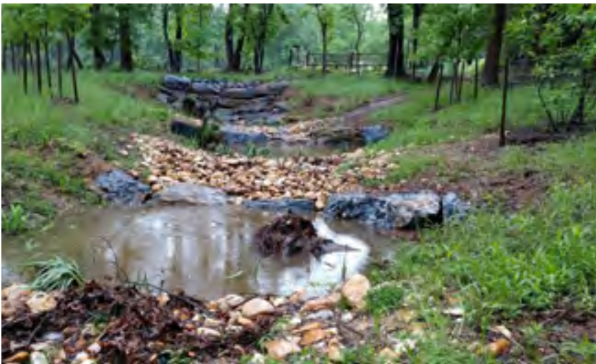
Step pools were installed in Dogwood Park to retain and slow water in a series of steps as water flows from an outfall into a tributary of Cabin John Creek. The project also restored highly eroded stream banks. Slowing and retaining water behind the steps reduces the flash speed of runoff when it rains, which helps to protect banks from future erosion.
