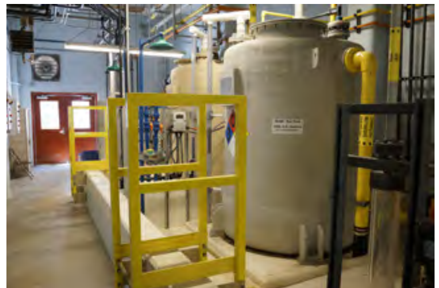
Rockville operations staff at the City's Water Treatment Plant (top); Water Treatment Plant equipment (bottom)
