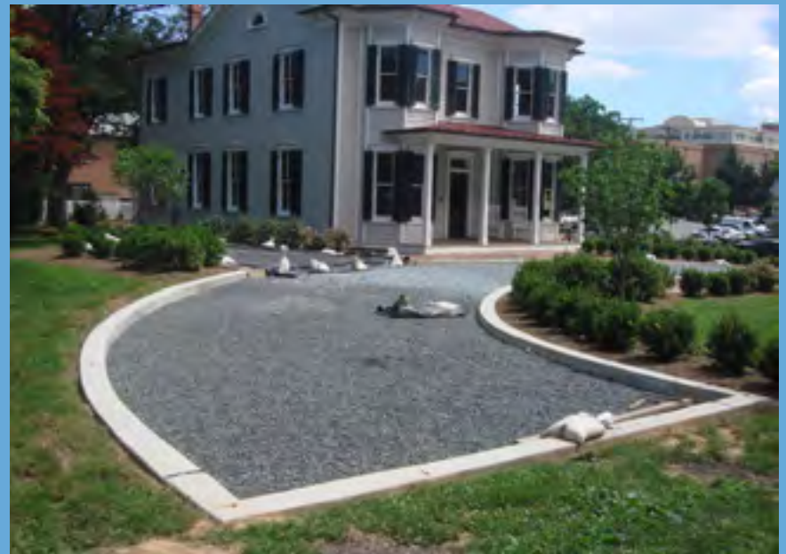
An historic house on West Jefferson Street installed a permeable paver driveway in 2018, shown here during construction of the gravel subsurface.
